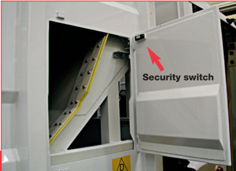
✓ Lockable access door with security switch
