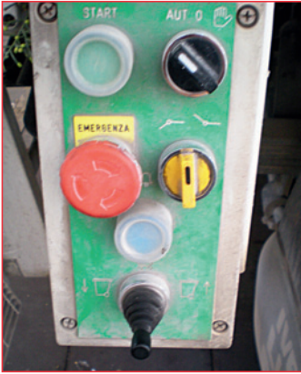
X Control panel unprotected against unintended actuation
