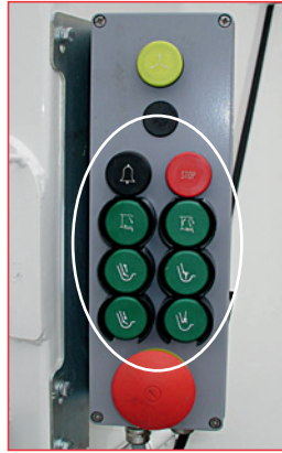
✓ Control panel with buttons protected against unintended actuation
